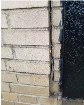
25) Vertical debonding of mortar at column.
