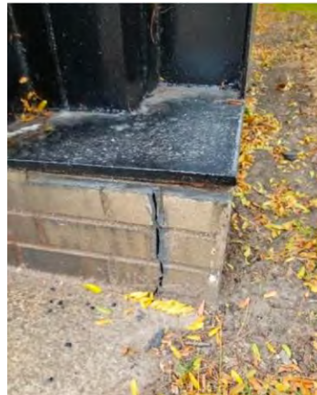
26) Vertical foundation crack.
